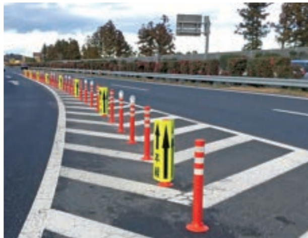
Countermeasures for wrong-way driving at a ramp merging section
