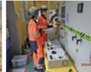
Inspection of a power substation
